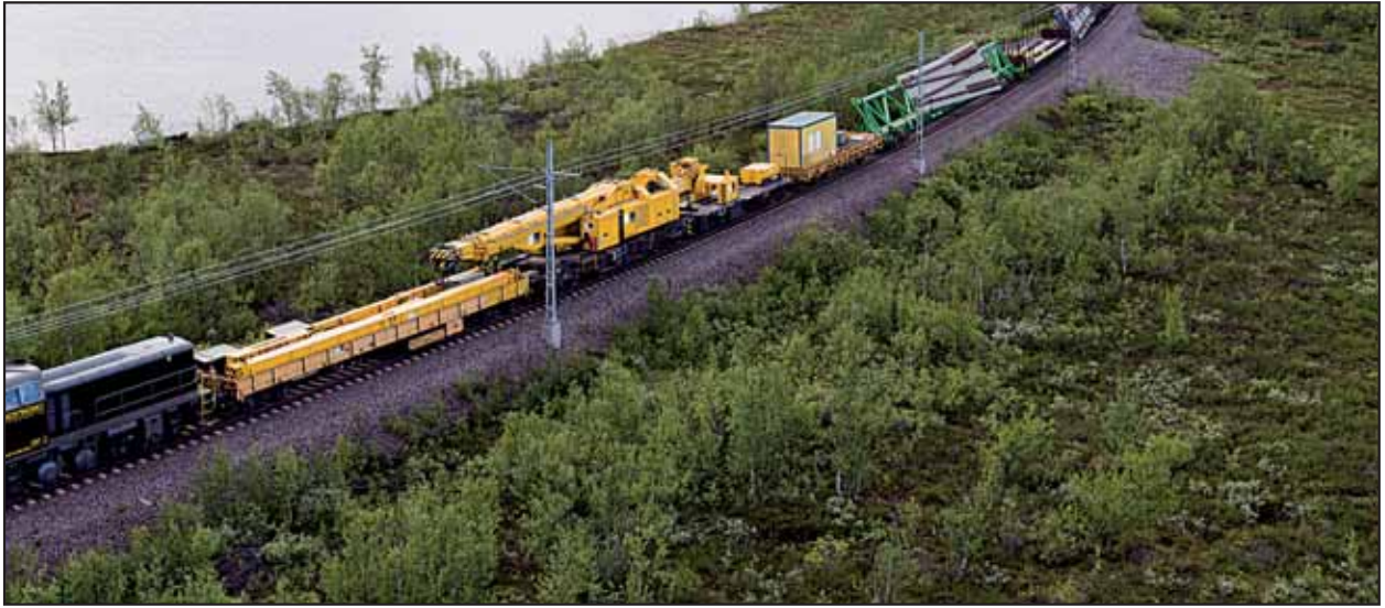
In Sweden, exchanging a turnout only takes eight hours, as Vossloh manufactures turnouts on site that are transported in pre-assembled segments on their own turnout carrier wagons before they are installed on site. Moreover, the Group is in charge of maintenance and servicing over the entire life cycle.
