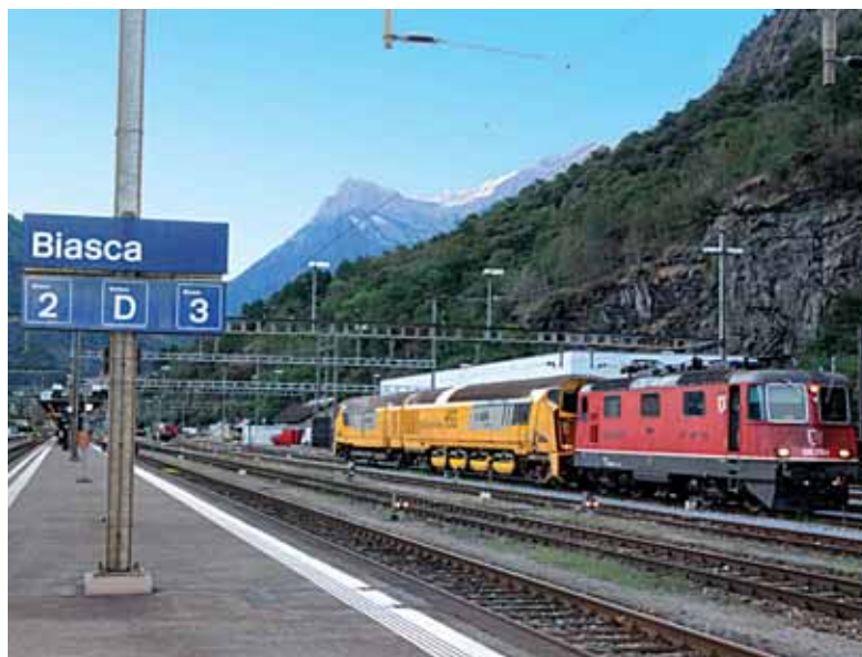
Since October 2016, grinding campaigns have been taking place on a regular basis in the Gotthard Base Tunnel to maintain the infrastructure in the world's longest railway tunnel.
