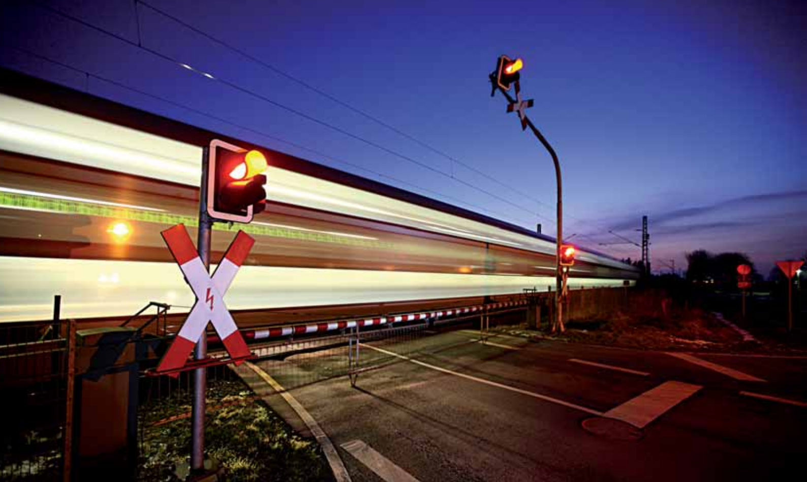
Level crossing “Schwarzer Weg” at the Oberhausen–Emmerich route. The signal system was designed by PINTSCH BAMAG.
